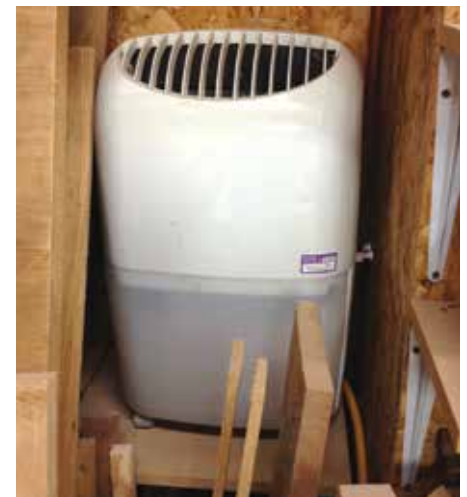
Our plumbed-in dehumidifier drying the timber
